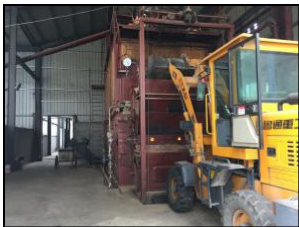
10t/h 蒸汽锅炉
