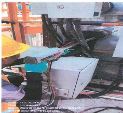
DA001 粉尘排气筒
